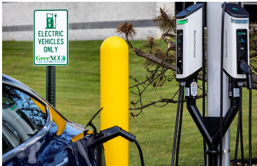
Electric Charging Station located at the Government Center
